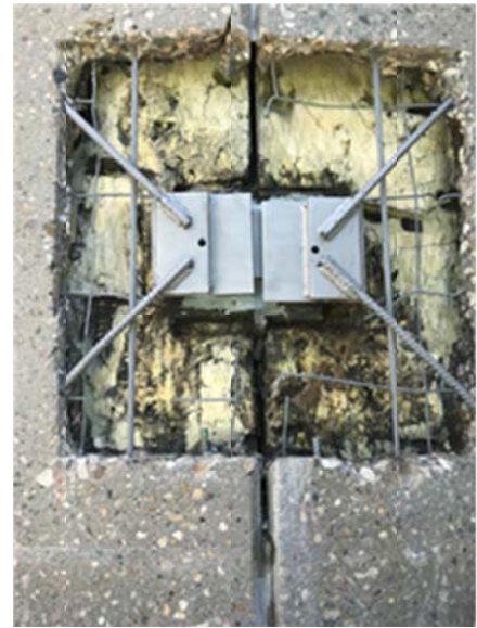
Structural weld plates that connect adjacent pre-cast concrete panels are being cleaned and inspected.
