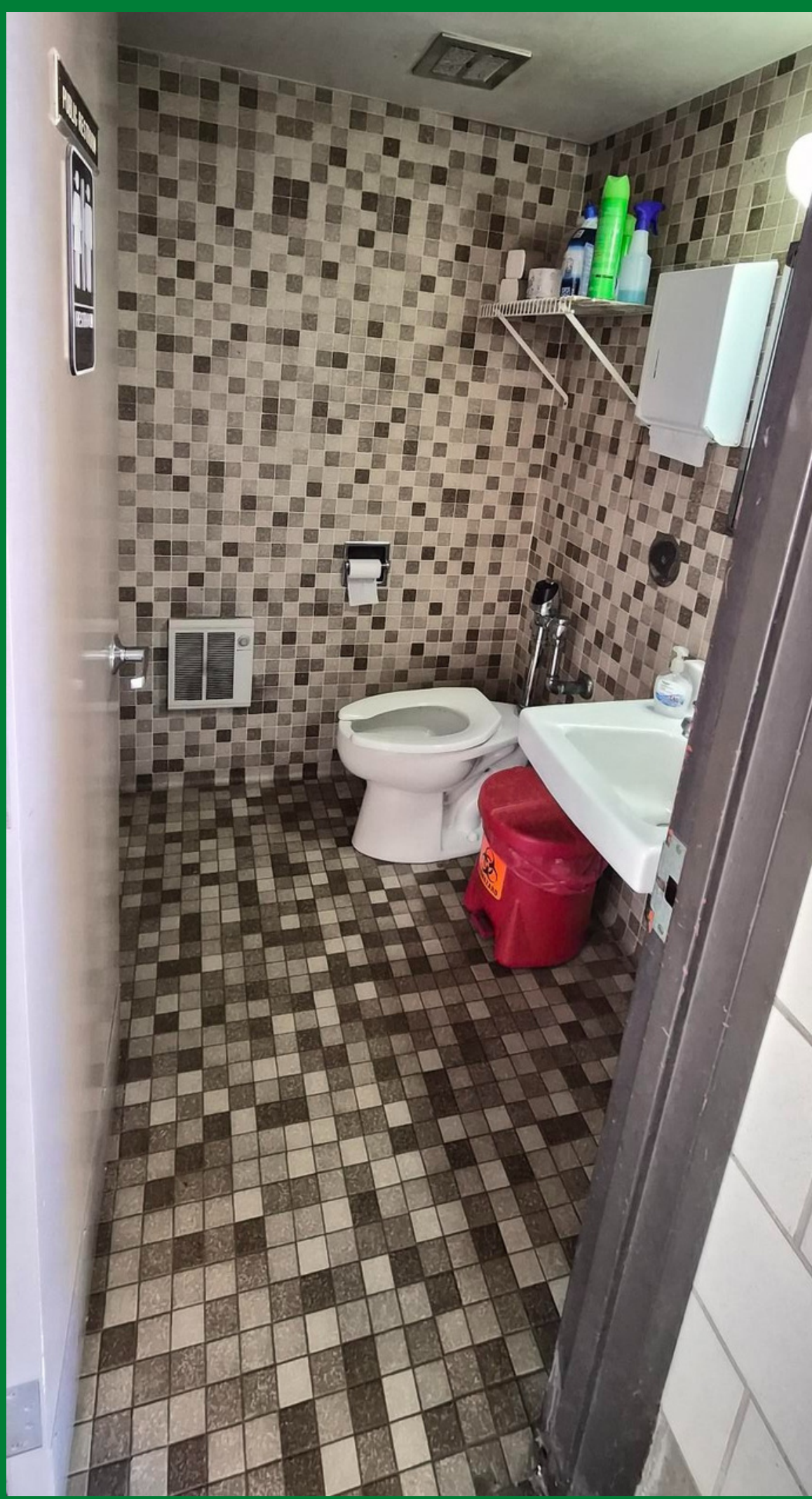
Decon bathroom does not have a shower
