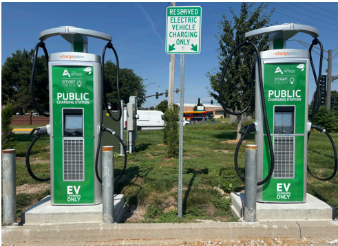
New Level 3 DC Fast Chargers were installed at 650 Lincoln Way.
