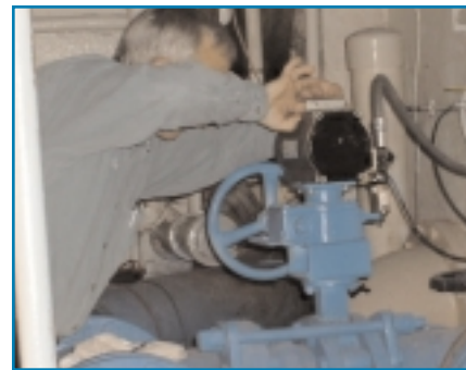
Checking a filter valve
